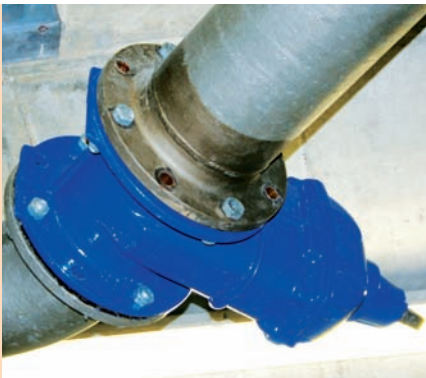
Figure 1 - Replacement of a gate valve with a ERHARD ROCO Premium dismantling type during inspection work on the state water supply of Baden-Württemberg.
